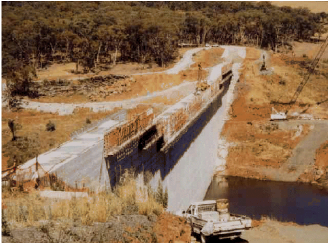
The Cadiangullong dam in Australia, constructed with Grout Enriched RCC facing. The surface is smooth and impervious.
