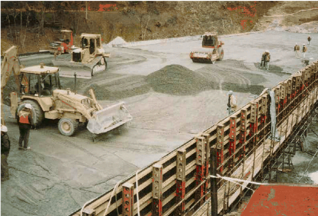
Above: Placement of the mortar layer between RCC lifts for Cadiangullong dam.
