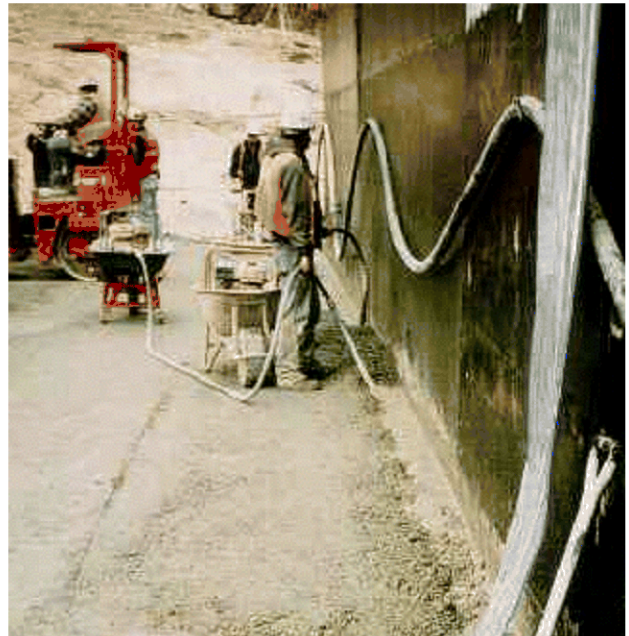
Above: Application of grout to facing RCC for GE-RCC. The facing RCC modified by grout and vibration can be seen against the forms,
